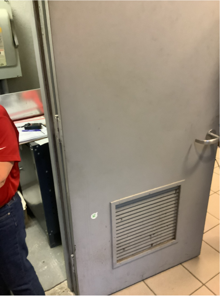
PHOTO #1 - ELEVATOR #3 - MACHINE ROOM
