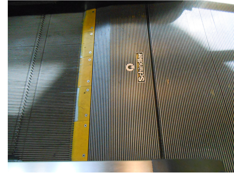
PHOTO #4 - ESCALATOR #4 - PIT COVER
