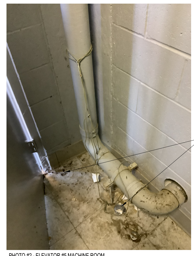
PHOTO #2 - ELEVATOR #5 MACHINE ROOM
