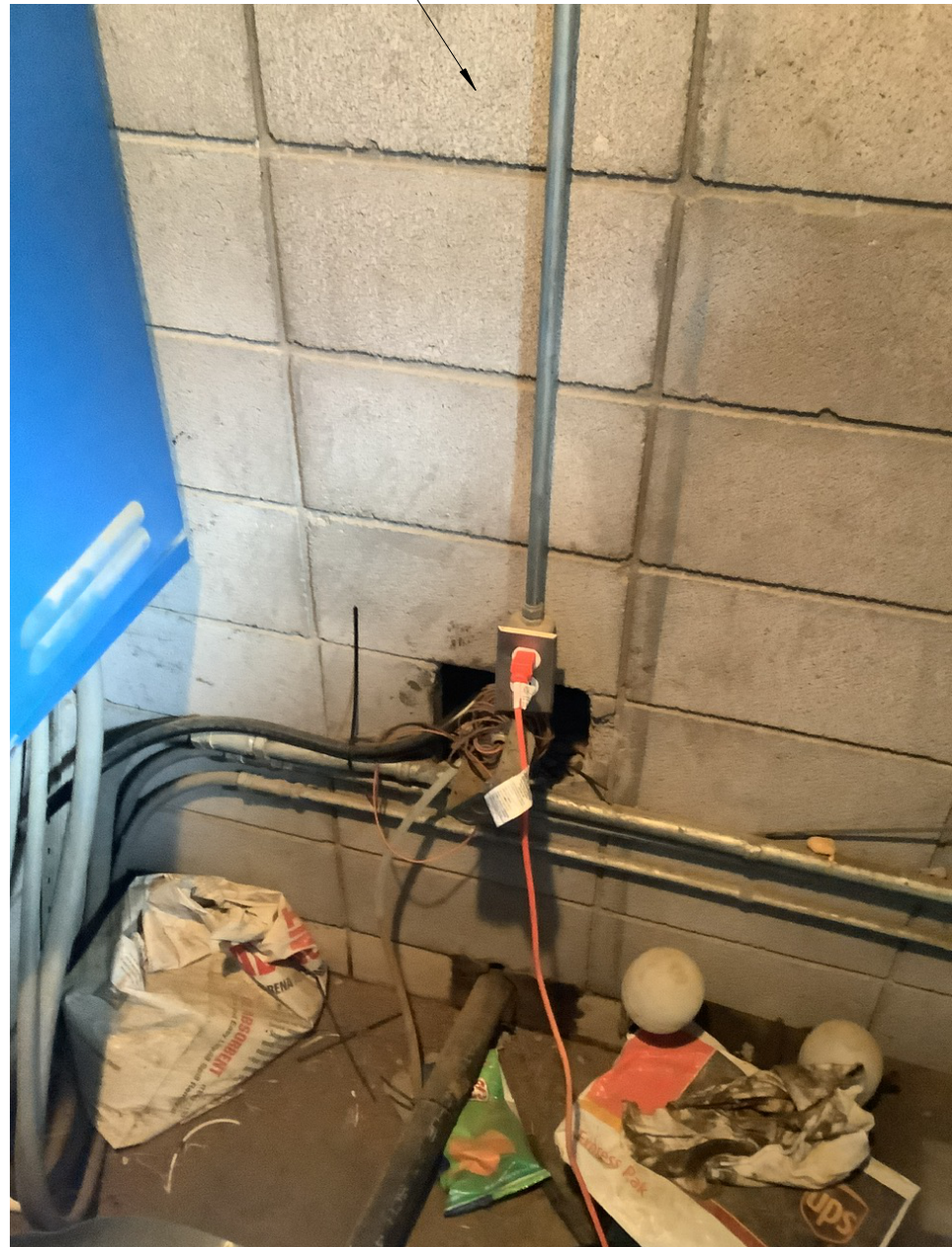
PHOTO #4 - ELEVATOR #2 - EXISTING ELEVATOR MACHINE ROOM
