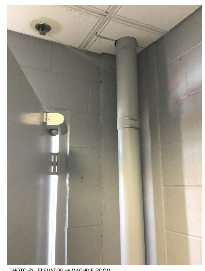
PHOTO #3 - ELEVATOR #5 MACHINE ROOM
