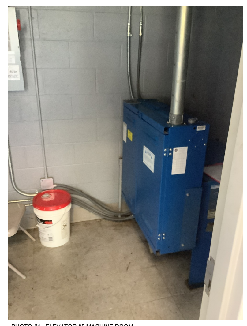
PHOTO #4 - ELEVATOR #5 MACHINE ROOM
