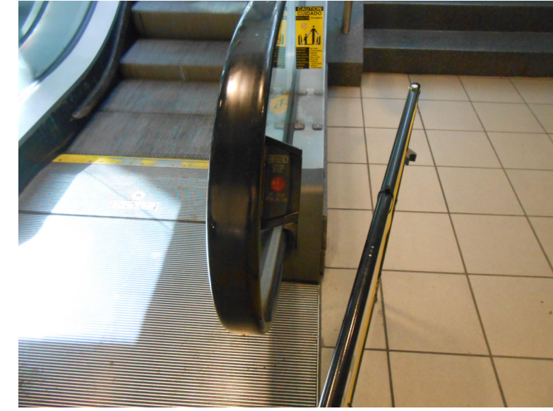
PHOTO #3 - ESCALATOR #4 - PIT COVER/ EMERGENCY STOP BUTTON
