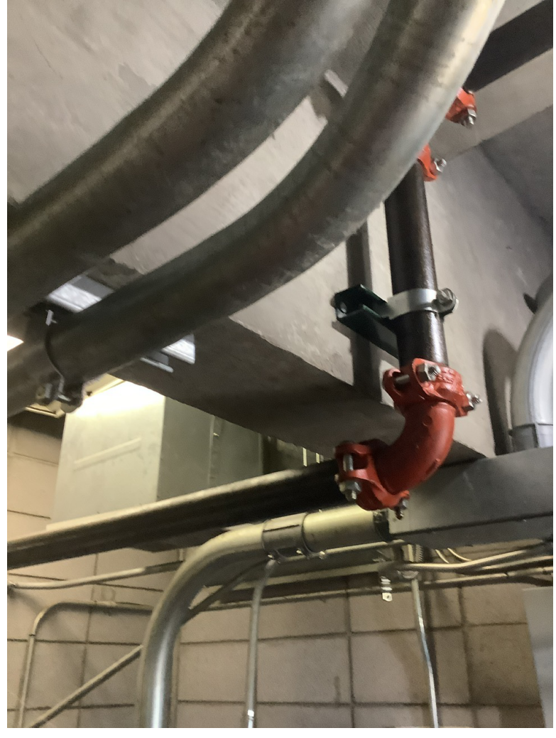
PHOTO #4 - ELEVATOR #4 - EXISTING PIPING IN MACHINE AREA
