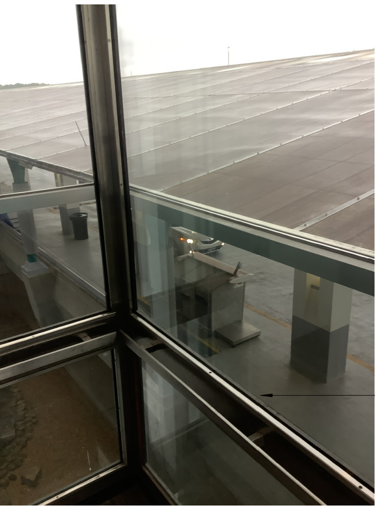
PHOTO #7 - ELEVATOR #3 - GLASS CABIN
